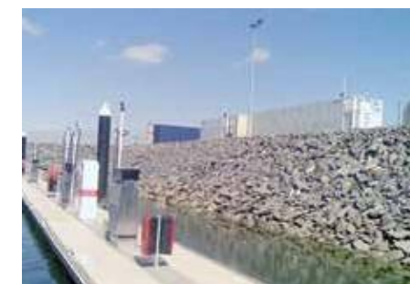
T80 & T30 : installed with floating pontoon for boat refuelling
