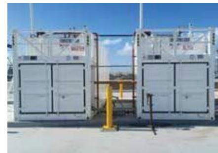
T30 : installed in master and slave
